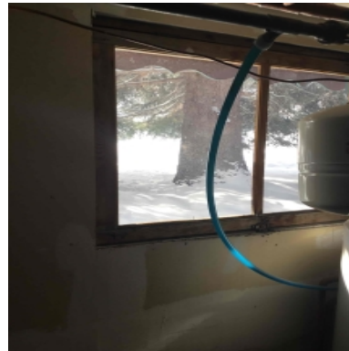
Single pane window with signs of deterioration .
