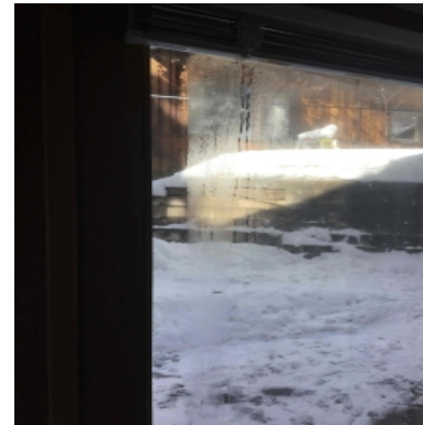
Double pane replacement doors with broken seals.
