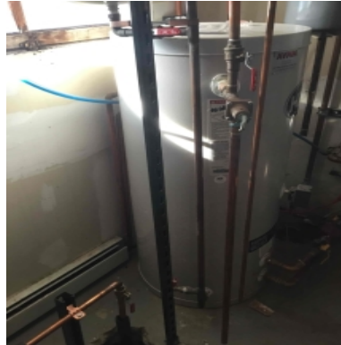
Sidearm DHW tank with uninsulated pipes .
