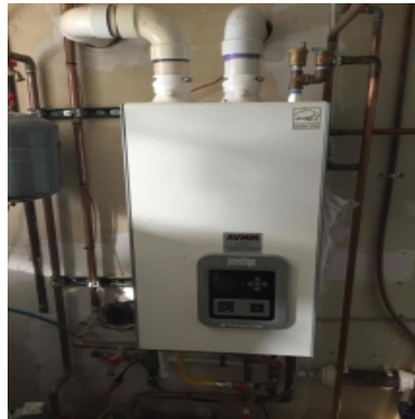
Sealed combustion gas boiler
