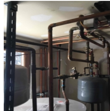
Uninsulated heat pipes
